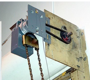
After replacing the traditional operating/closing system with an "Easy-Reset" retrofit fire door chain operator, the door now closes without a loss of spring tension. The door can now be reset by simply reconnecting the fusible link cable and opening the door (above).
