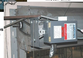
After retrofitting the fire door system is a simplified self contained system. Release mechanism and speed control governor are integrated into the motor unit.
